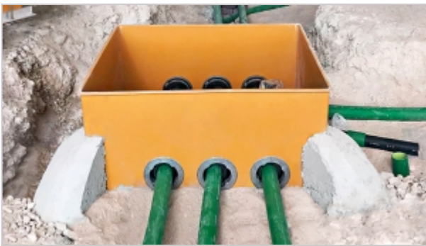
Vacuum testable Fibrelite GRP sumps provided a strong, hard-wearing, liquid-tight containment solution | © OPW Global
