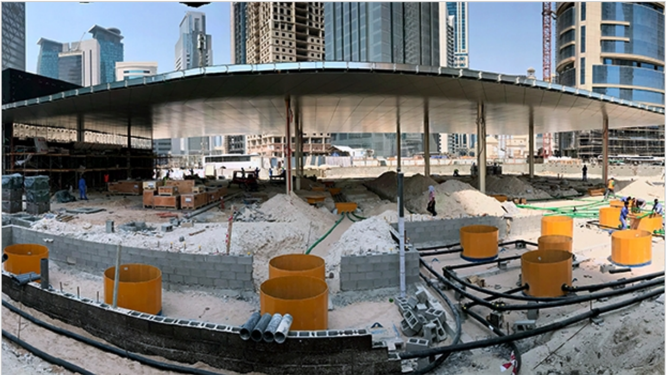
One of over 20 forecourt sites built during the first stage of the project | © OPW Global
