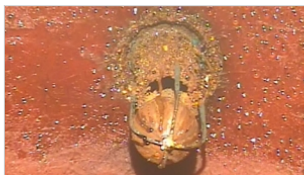
A severely corroded ball float inside a fiberglass tank
