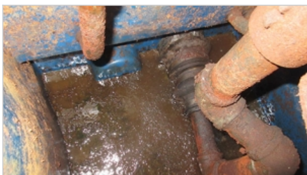
Sludge and corroded pipes in the Under Dispenser Containment
