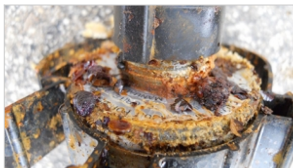
Corrosion deposits on the top of an ATG probe
