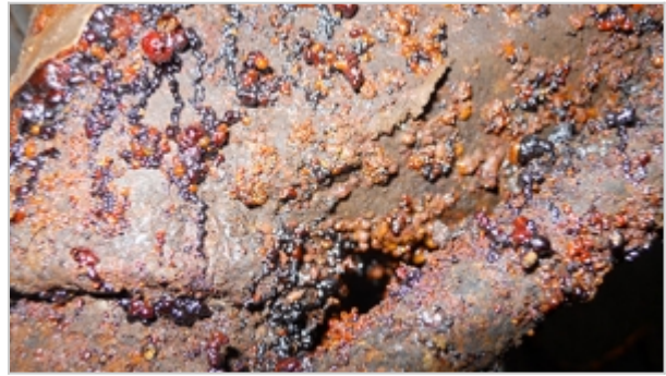
Corrosion and tubercles on the internal section of an STP
