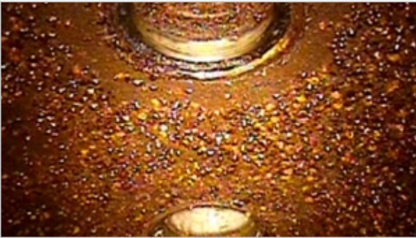
Internal view of corrosion inside a steel tank
