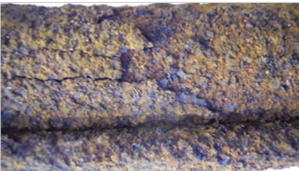
A severely corroded STP shaft that was removed from a diesel tank
