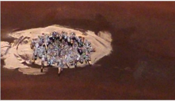
Severe corrosion and tubercles on a bung inside a fiberglass tank
