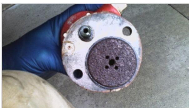
Corrosion on the functional element, a component of an STP
