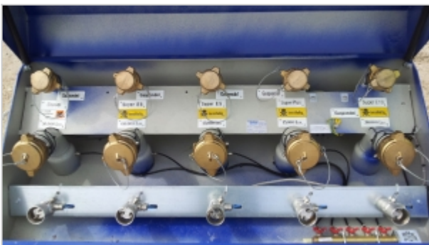
Cross-over-prevention and overfill prevention on a petrol-station filling point | © Secu-Tech
